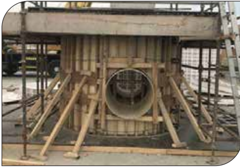
Manholes for Sewer and Drain
